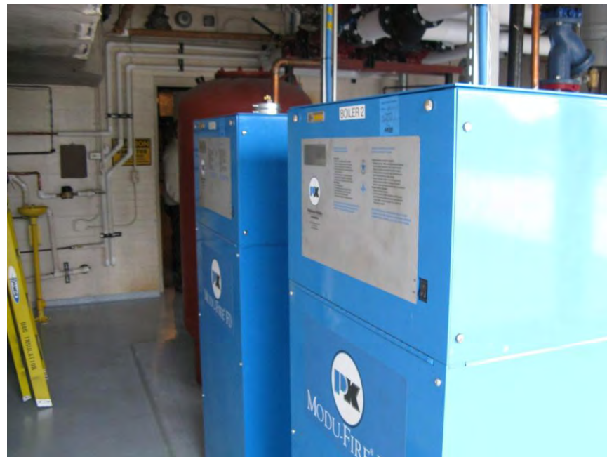
Boilers within Mechanical Room
