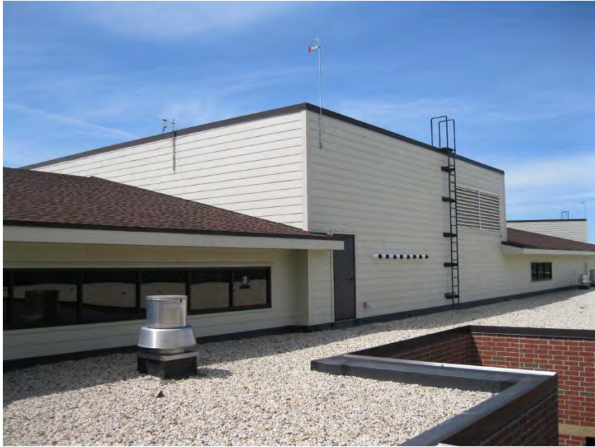
Exterior View of Upper Level Mechanical Area
