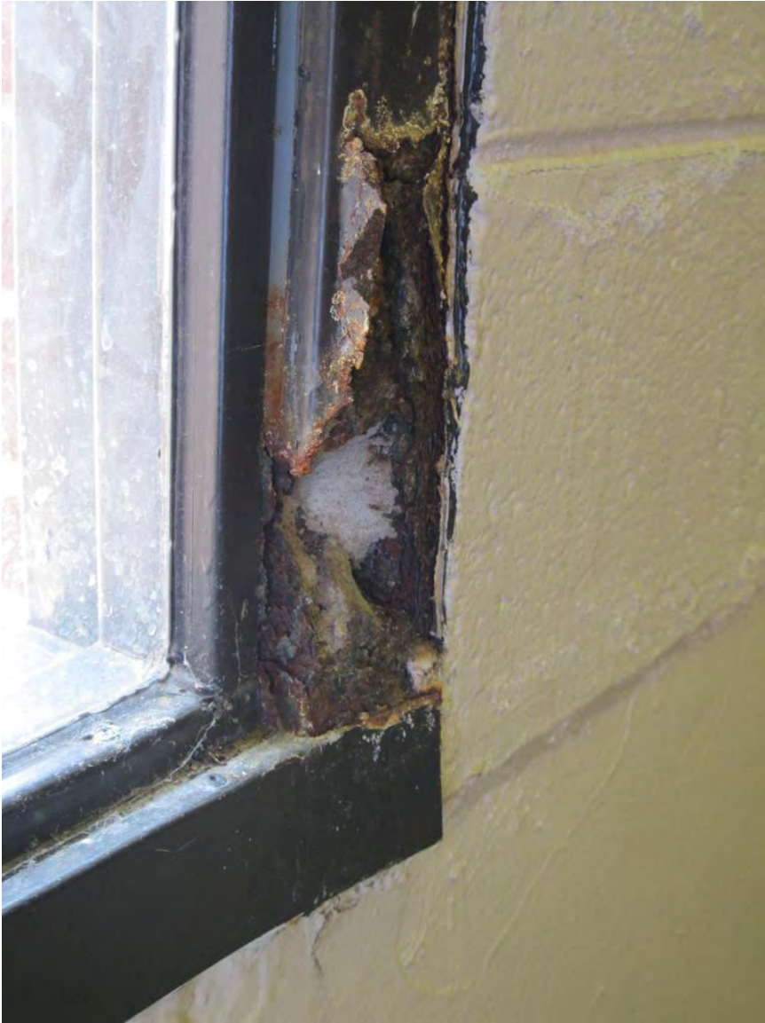
Deteriorated Window Frame
