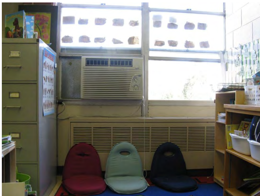
Classroom Air Conditioner and Unit Ventilator
