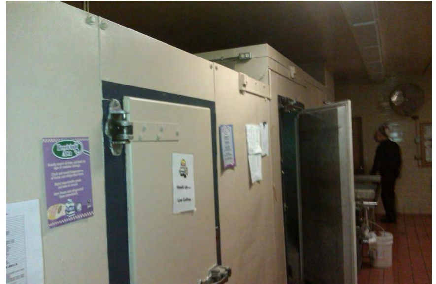
Kitchen Freezer & Cooler
