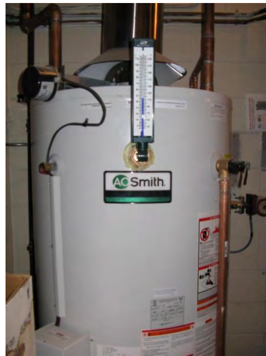
Hot Water Tank
