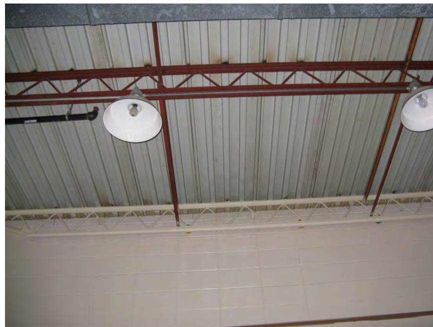
Assembly Hall Ceiling Showing Outdated Light Fixtures
