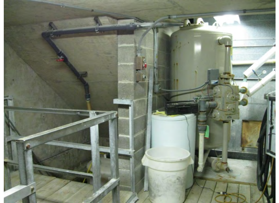
Pool Mechanical Room
