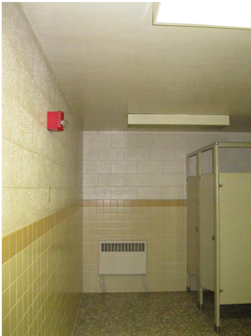
Typical Outdated Restroom
