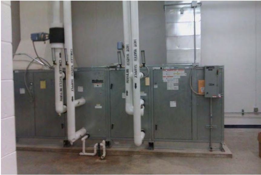
Typical Air Handling Unit
