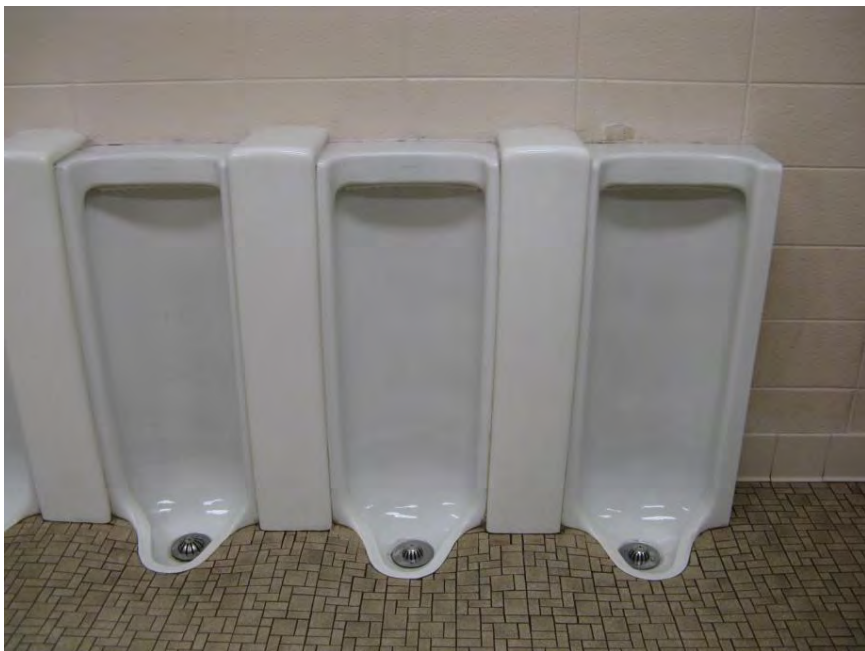
Outdated Men's Restroom
